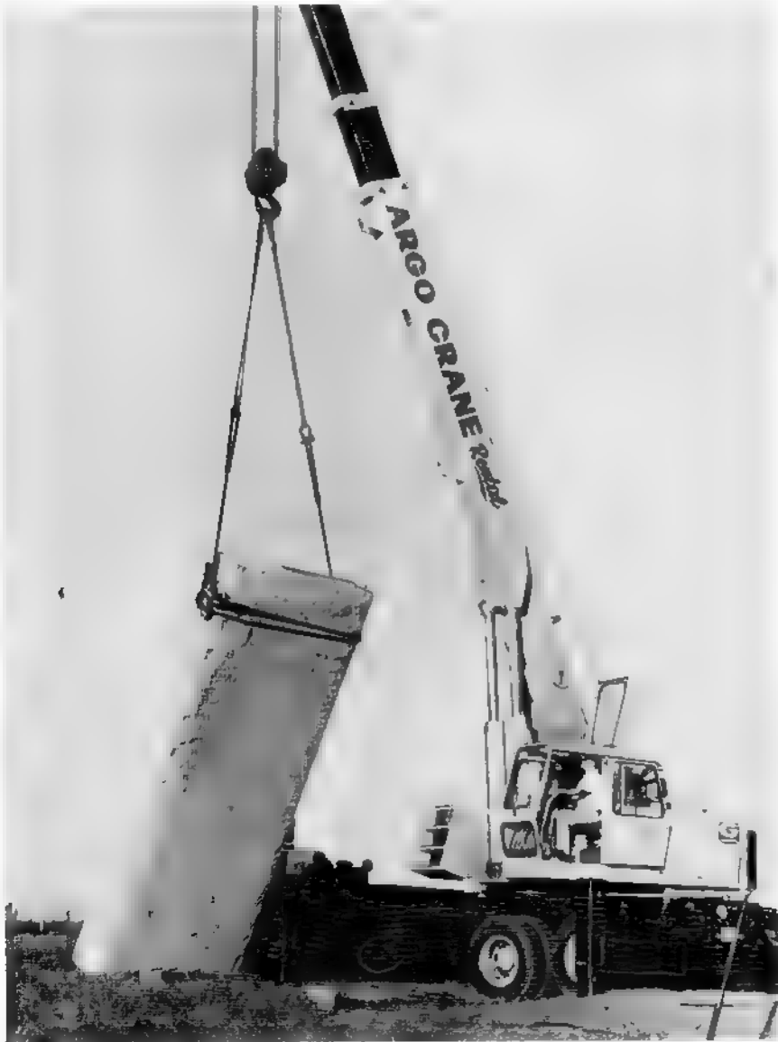
With ultimate precision and true dedication, Grady H. Albertson, owner and operator of Argo Crane Company handled the erection of 'The Georgia Guidestones'. He is shown lifting the first Guidestone to its final resting place.
